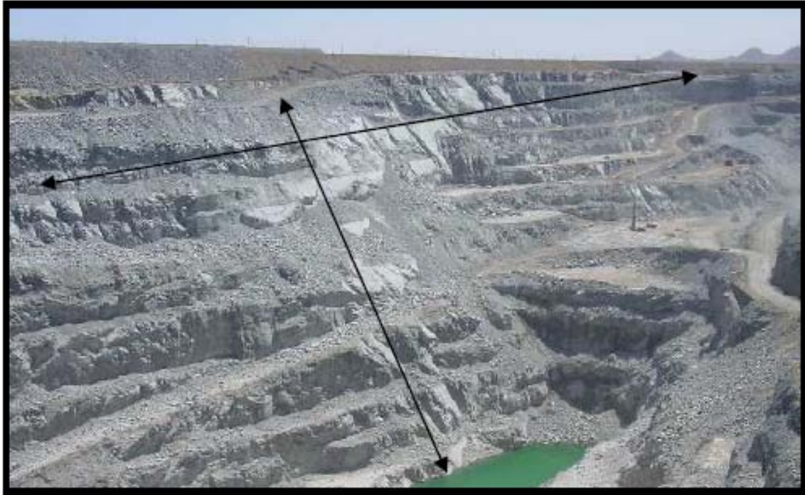
Figure 3 Photograph of fault zones cross-cutting the west wall of Sandsloot open pit.
